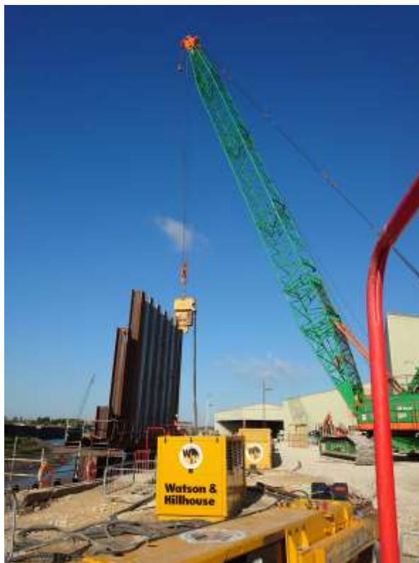
Plate 2-18: An example of a crawler crane, used to drive sheet piles (photo provided by BAM Nuttall Ltd)
