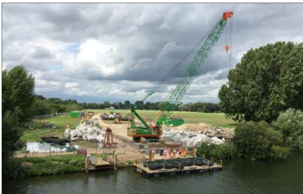
Plate 2-19: An example of a temporary wharf (photo provided by BAM Nuttall Ltd)
