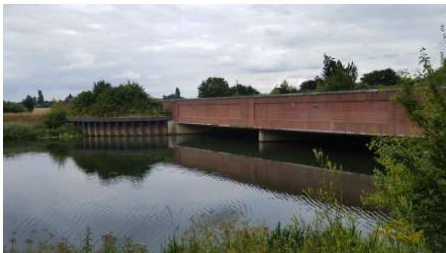
Plate 2-8: An example of a typical road bridge for the flood channel to pass underneath.
